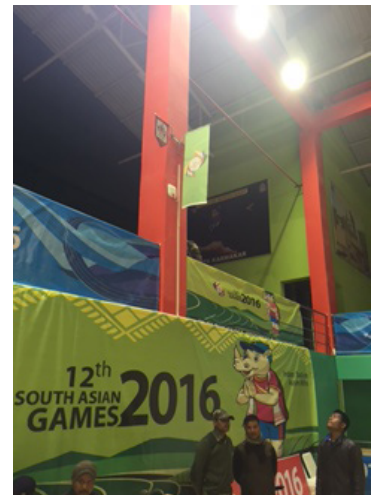
cnPilot enterprise access point installed indoors
